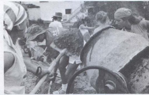
BUILDING THE ROAD IN KIRNI TOOK DETERMINATION, EFFORT AND SEVERAL TONS OF CEMENT, SEEN HERE BEING MIXED BY A GREEK SUMMER PARTICIPANT.
