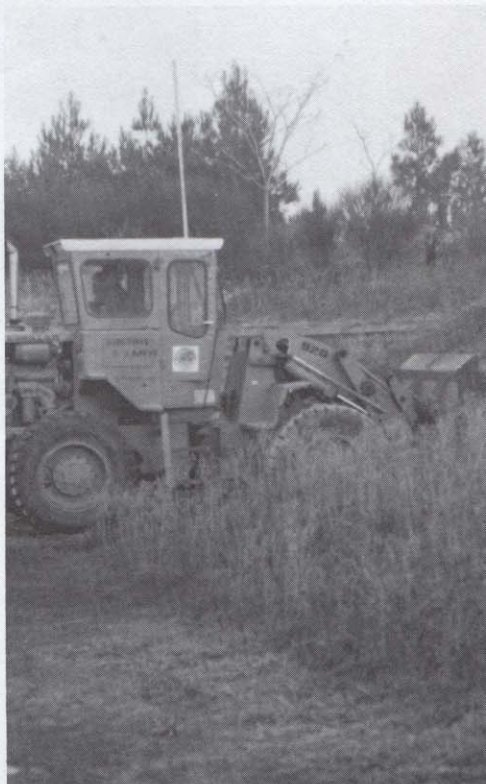
The first "shovel full" of earth is removed for the construction of the Henry R. Labouisse Youth Recreation Center.
